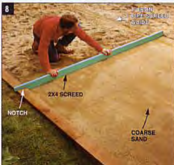
8 1" IRON 3" PIPE SCREEN GUIDE 2X4 SCREED NOTCH COARSE SAND SPREAD AND LEVEL a 1-in. bed of sand over compacted subbase. Pipes provide a guide for dragging the 2x4 screed board across.
