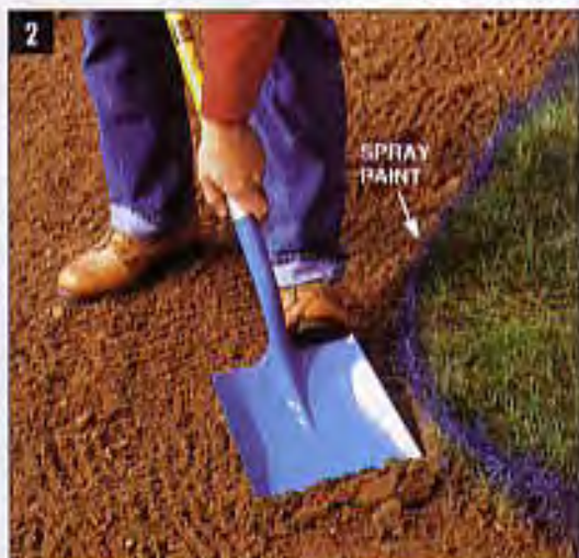
REMOVE SOD in an area extending 8 in. beyond the boundaries of the patio. Spray paint indicates the excavation line.
