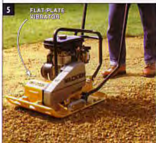
5 FLAT-PLATE VIBRATOR TAMP THE SUBBASE using a flat-plate vibrator (rented at $40 a day). Work in a circular motion and compact the area twice.
