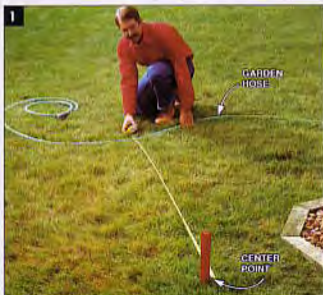
OUTLINE the patio perimeter using a garden hose for curved areas and long 2x4s for straight sections.
